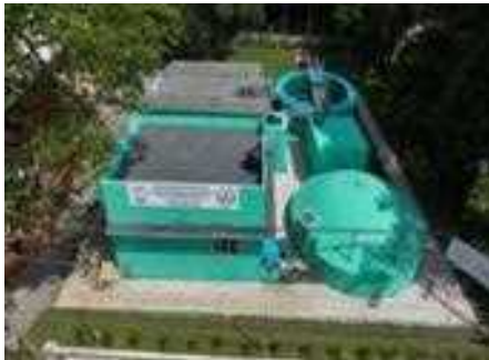
360 KLD STP at General Hospital, Thrissur
