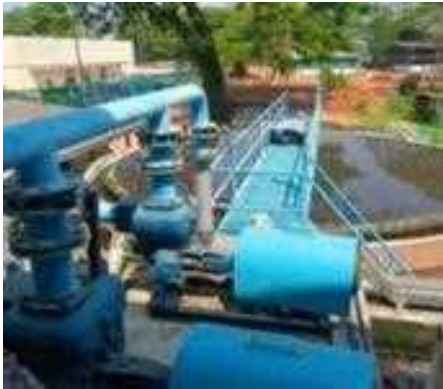
500 KLD STP at Kozhikode medical College
